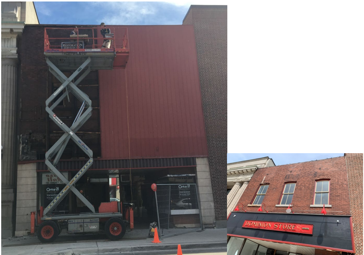
Figure 1: Newer materials covering traditional façades should be removed where possible, and original building features should be restored.
