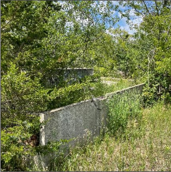
Image 9 : Concrete footings and disturbance.
