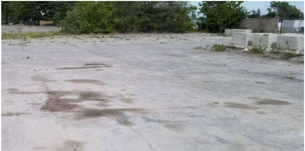
Photo 8: The eastern Hydrocarbon staining (PCA 28) observed within the foundation of the main building looking east
