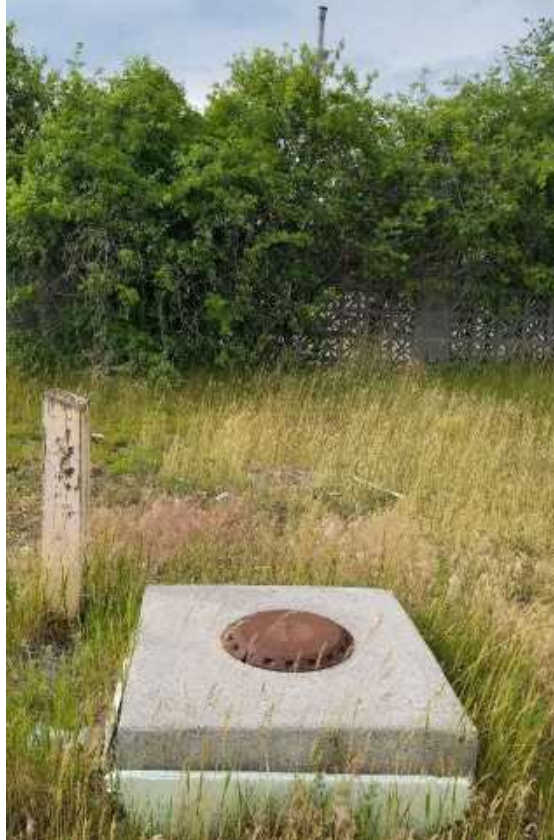
Photo 3: Fill cap for UST (PCA 28) buried in the eastern portion of the Phase One Property looking north towards the ventilation pipe located along the wall
