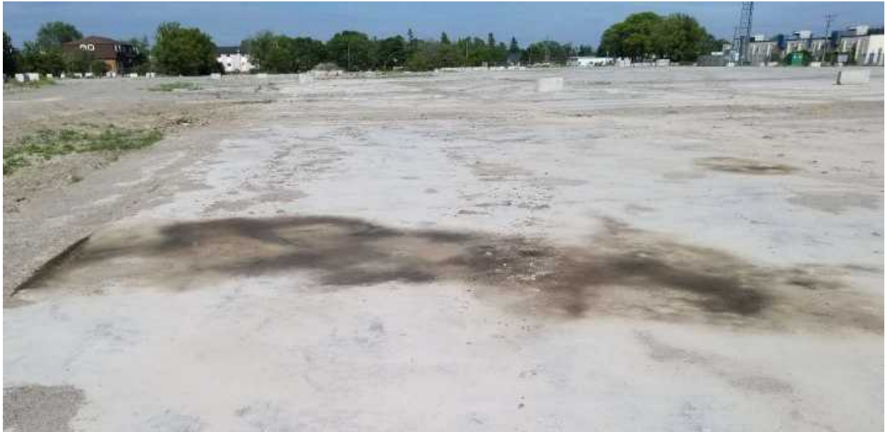
Photo 7: The western Hydrocarbon staining (PCA 28) observed within the foundation of the main building looking east
