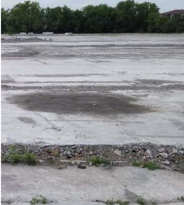
Photo 9: The central Hydrocarbon staining (PCA 28) observed within the foundation of the main building looking north
