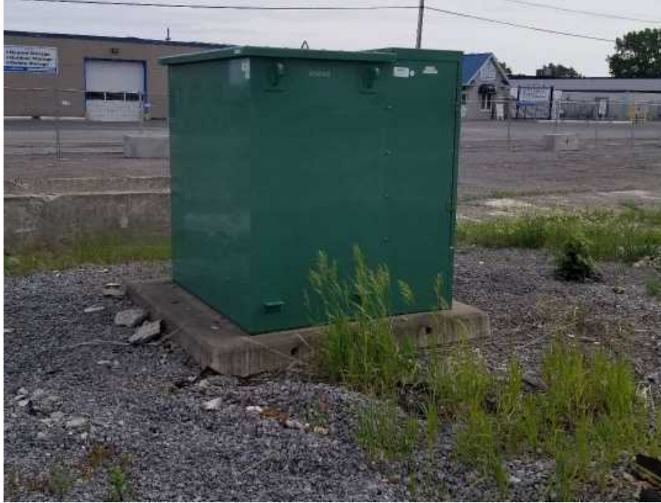
Photo 5: Electrical transformer (PCA 55) located on the Phase One Property just to the south of the main building
