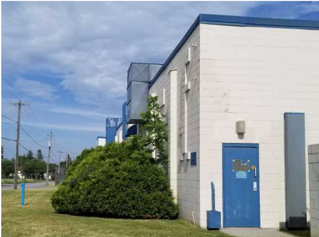
Photo 20: Two monitoring wells present at 35 Wilson Avenue with distribution transformer (PCA 55) in the background looking towards the east
