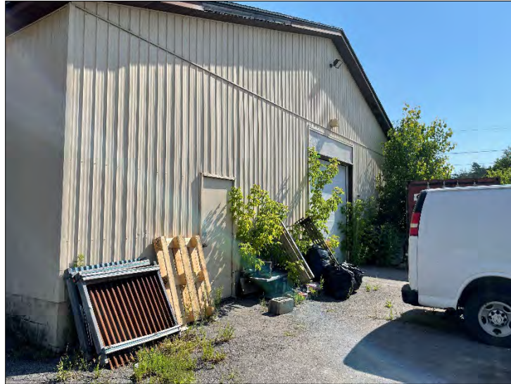
Front View of subject property at 84 Cannifton Road N main building. Picture taken facing east from west side of the Site.
